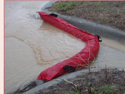
1 "Big Red" CI protector protecting a concrete swale.
