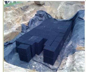
Infiltration tanks being installed under a geotextile layer. This 2500 gallon storage volume was installed in one day with a crew of 4.
