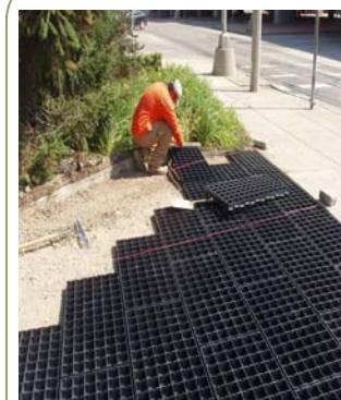
Geoblock 5150 (Grass Pavers) Ideal Landscape Group employee Installing product after sub-grade was prepared
